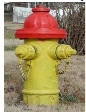
Older Fire Hydrant
